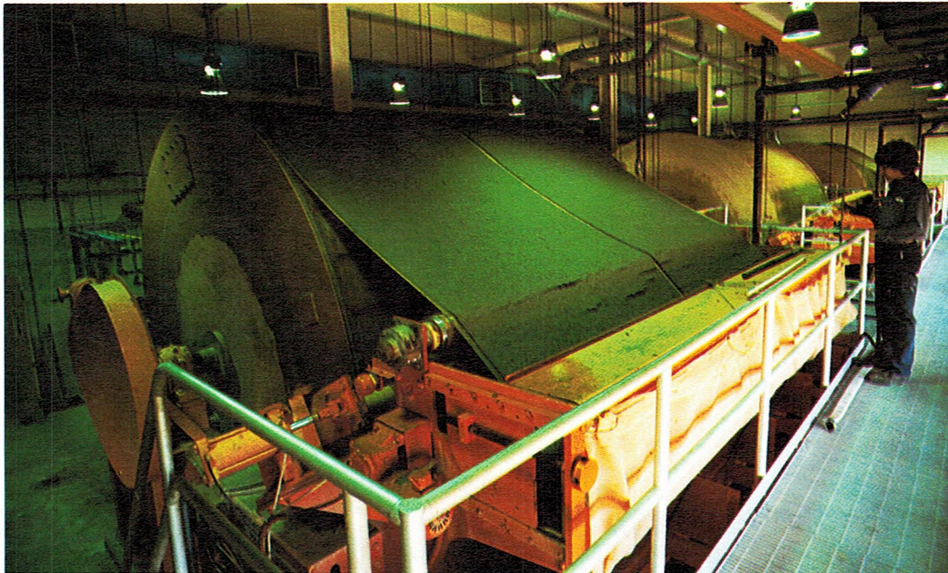
Sludge Dewatering Filter System
